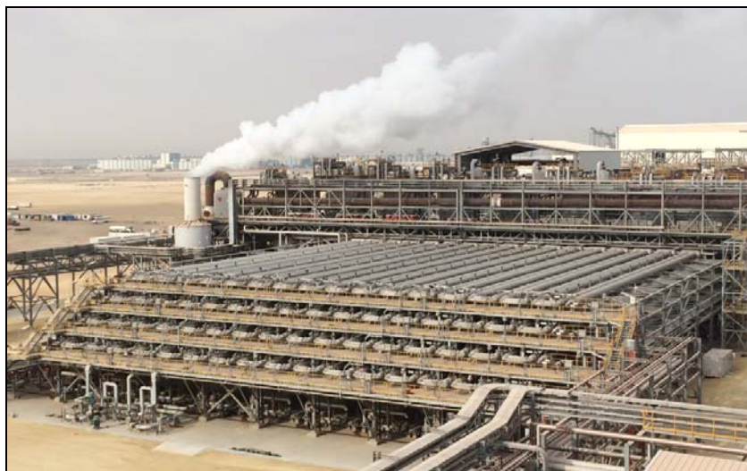
Figure 2. Digestion jacketed pipe heaters.
